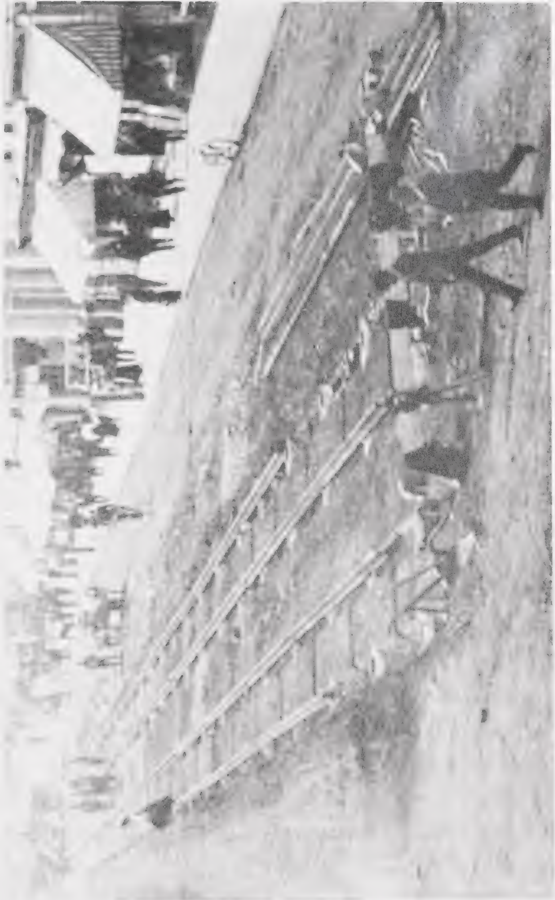
Plate 2. (City of Edmonton Archives) First Stages of Permanent Construction on Jasper Avenue, 1908
